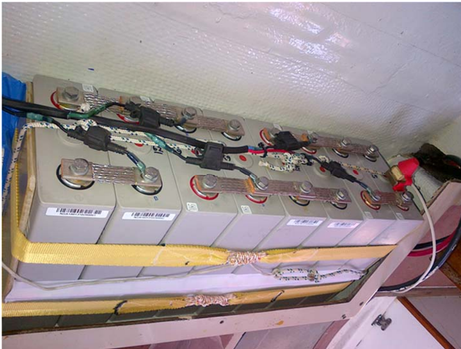
Cell layout and busbar configuration. The small wires are for the BMS. They have 1 amp fuses in waterproof holders. The temperature cutouts are underneath the white insignia cloth visible between the two Kevlar straps. The terminal fuse is visible on the positive end of the bank.
