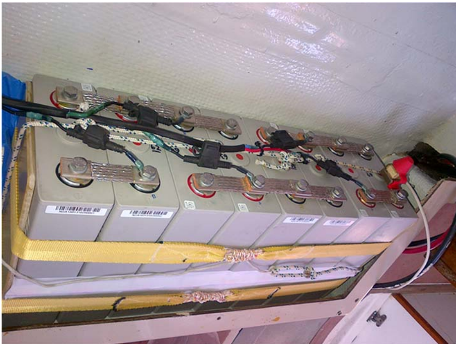
Cell layout and busbar configuration. The small wires are for the BMS. They have 1 amp fuses in waterproof holders. The temperature cutouts are underneath the white insignia cloth visible between the two Kevlar straps. The terminal fuse is visible on the positive end of the bank.
